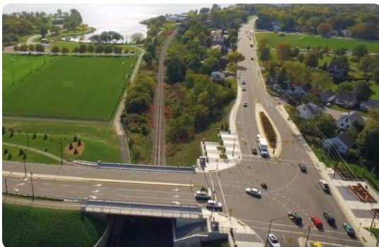
Rehabilitation of Baybridge Road CPR Overhead Bridge in the City of Belleville.
