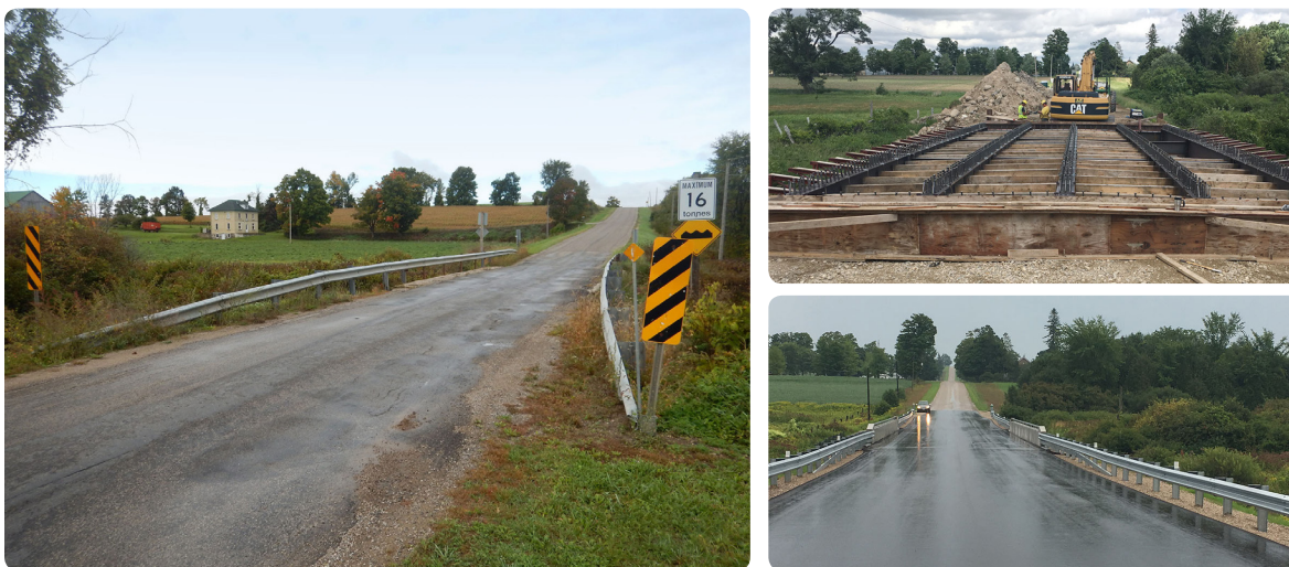
The Donaldson Bridge in the Town of South Bruce before (left) during (top right) and after (bottom right) replacement.
